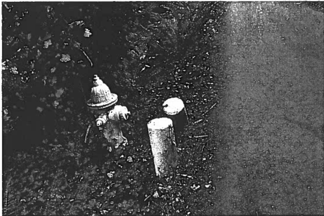
8. Leaning fire hydrant along shared access road.
